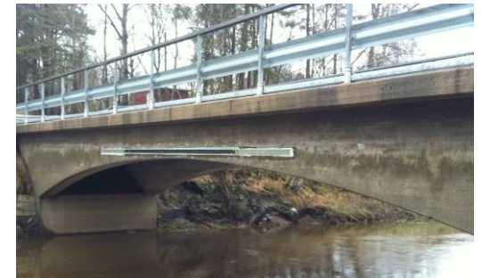
Strengthening of Nossan Bridge using pre-stressed CFRP laminates in collaboration with Swedish Transport Administration
