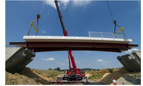
Application of FRP composites in bridges: Installation of a light weight hybrid FRP bridge in Germany.
