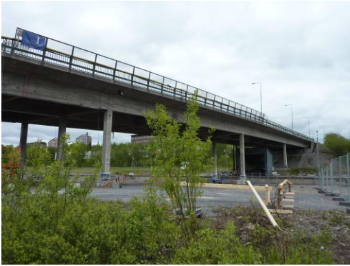
Strengthening of gruvvägen bridge in Kiruna in Collaboration with Swedish Transport Administration and LTU
